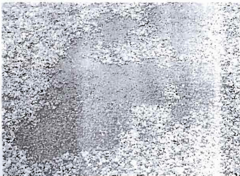
Photo 32 Arrachement discontinu type plumage.
