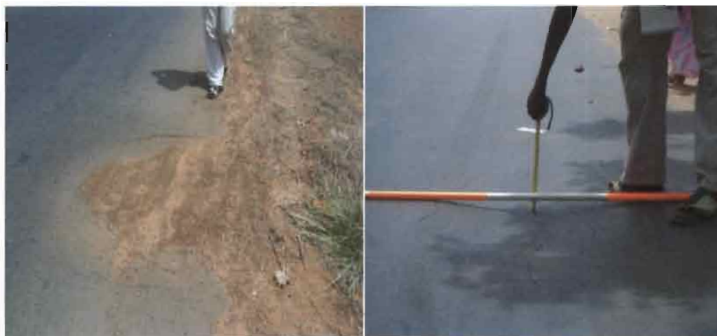
Figure III.2: Affaissement de rive (Route Notto-bayakh) Figure III.3: Affaissement hors rives (RN2)
