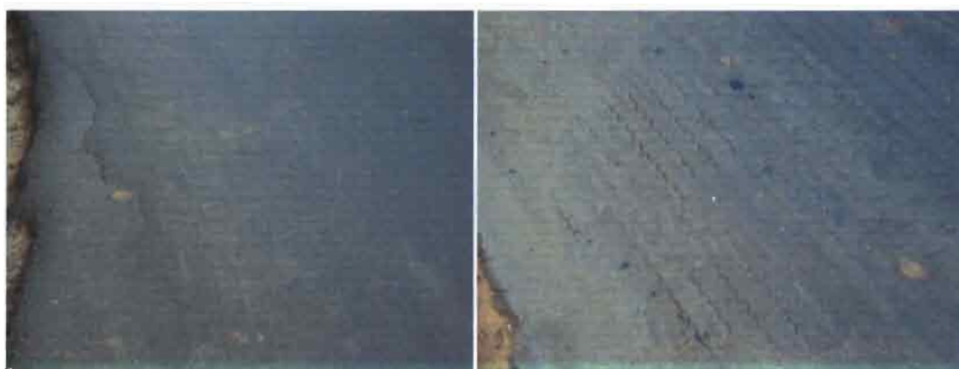
Figure III.27: Ressuage sur la RN3
